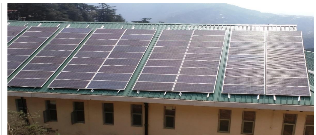
Solar Energy Panels installed in Administrative Block of the High Court of Himachal Pradesh
